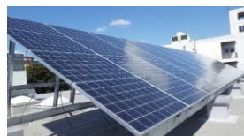
Solar power generation
